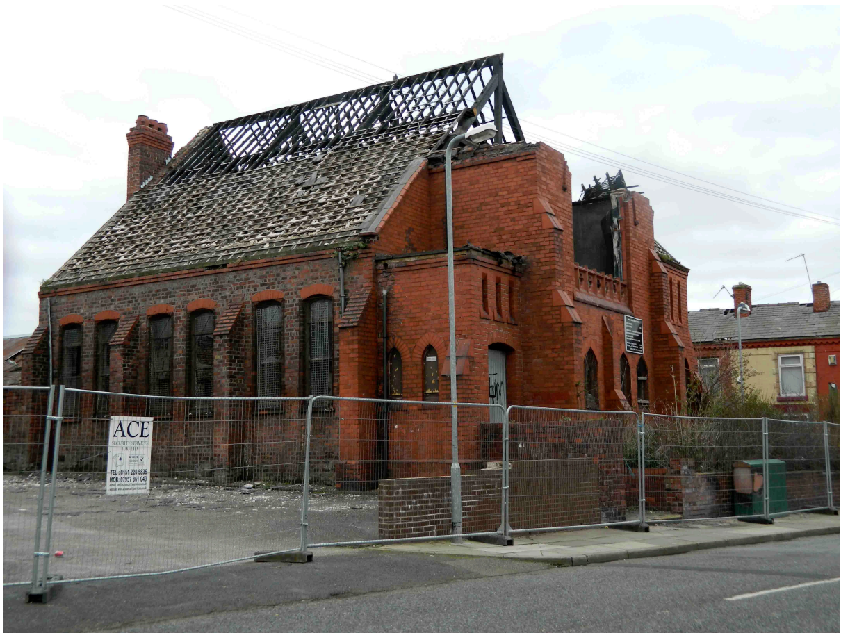
Springwell Chapel, Klondyke, Liverpool, partially demolished.
